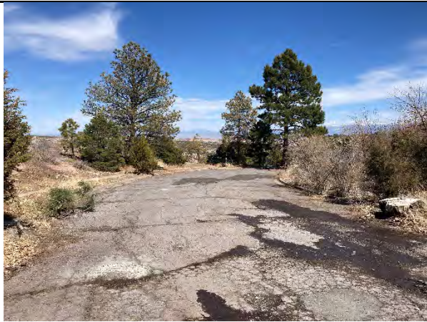
Barranca Rd walkup and undefined parking area
